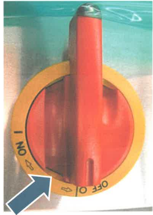
New switch lockout location
